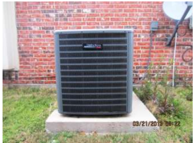
Picture #11 AC Unit
