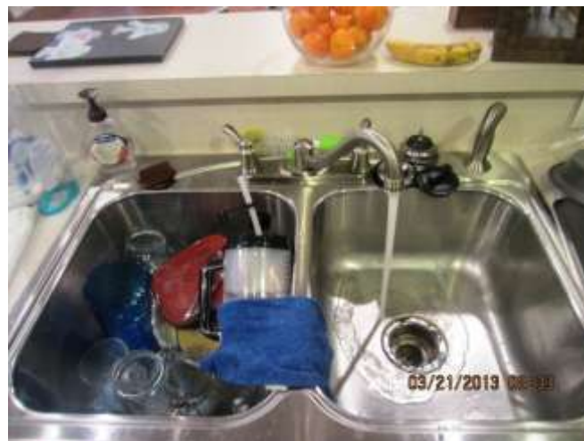
Picture #48 Sink Faucet/Back Splash
