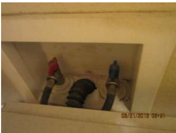
Picture #98 Washer Connection
