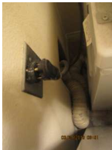
Picture #99 Dryer Vent
