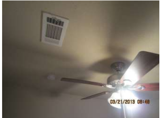
Picture #76 3 rd Ceiling/Light/Fan/Smoke Detector
