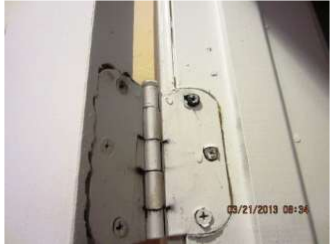
Picture #52 Loose Hinge
