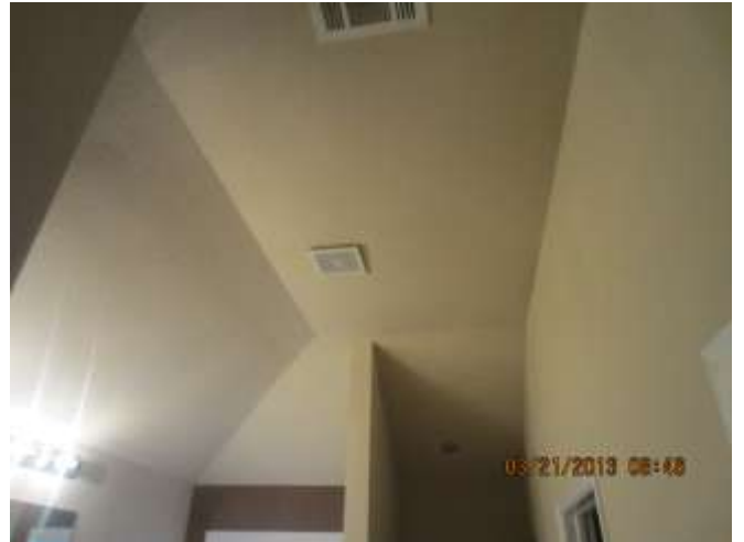
Picture #66 Bathroom Ceiling
