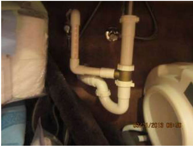
Picture #85 Cabinets Interior/Shut-off valves
