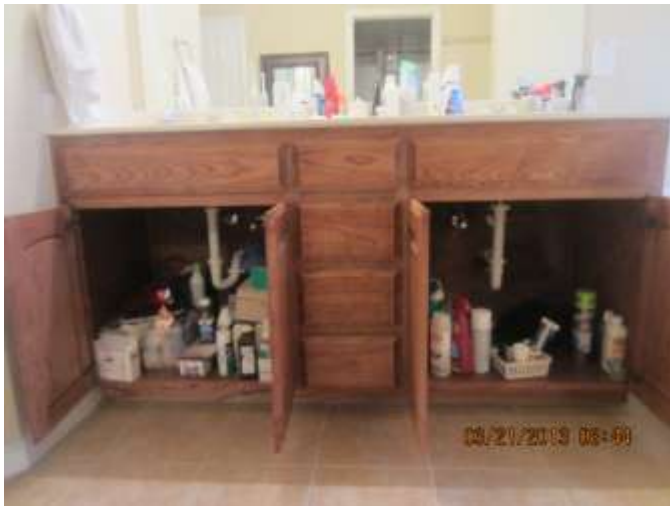
Picture #63 Cabinet Interior/Shut-off valves
