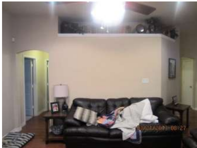
Picture #27 Living Room Wall
