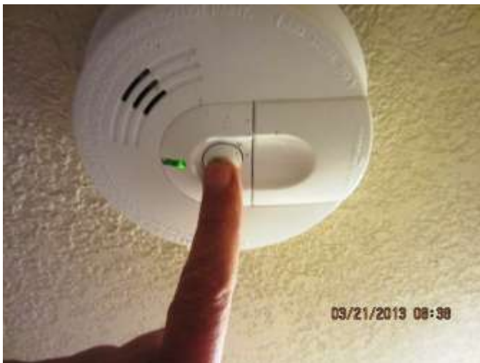
Picture #70 Smoke Detector
