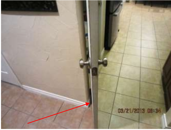
Picture #51 Any Concerns (Missing Door Stop)
