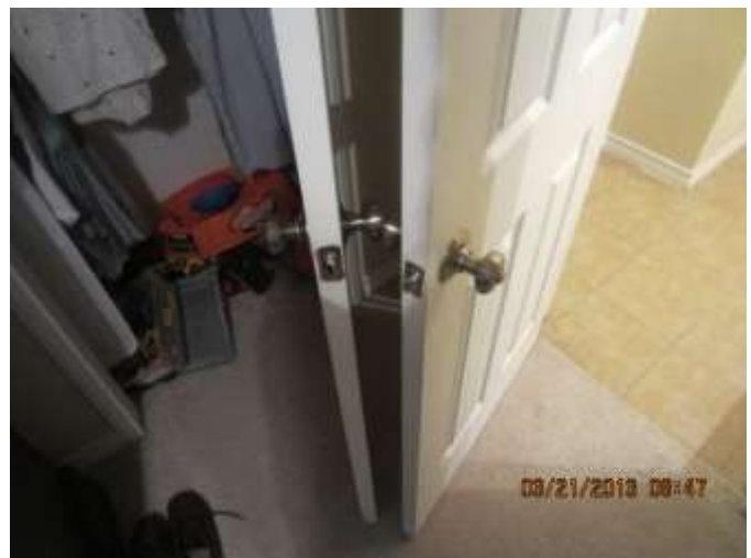
Picture # 74 Missing Door Stops
